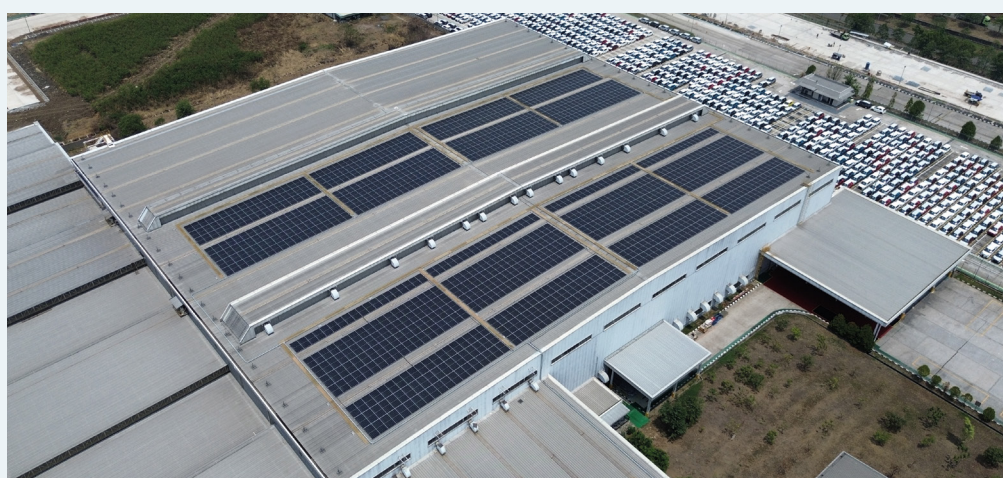
Solar panels at PT Astra Daihatsu Motor
