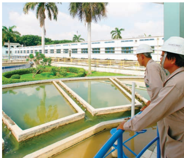
Water treatment plant Indonesia
